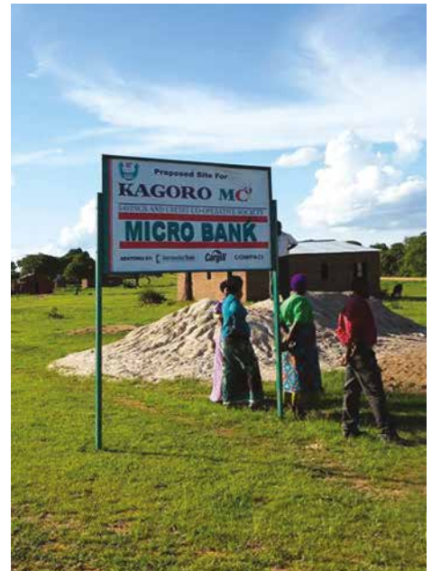
Building and river sand collected by the community for the construction at KABORO MC 2 (Zambia).
